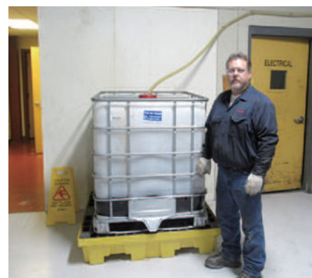
Waste oil recycling system
