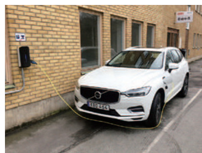
Power charging station
